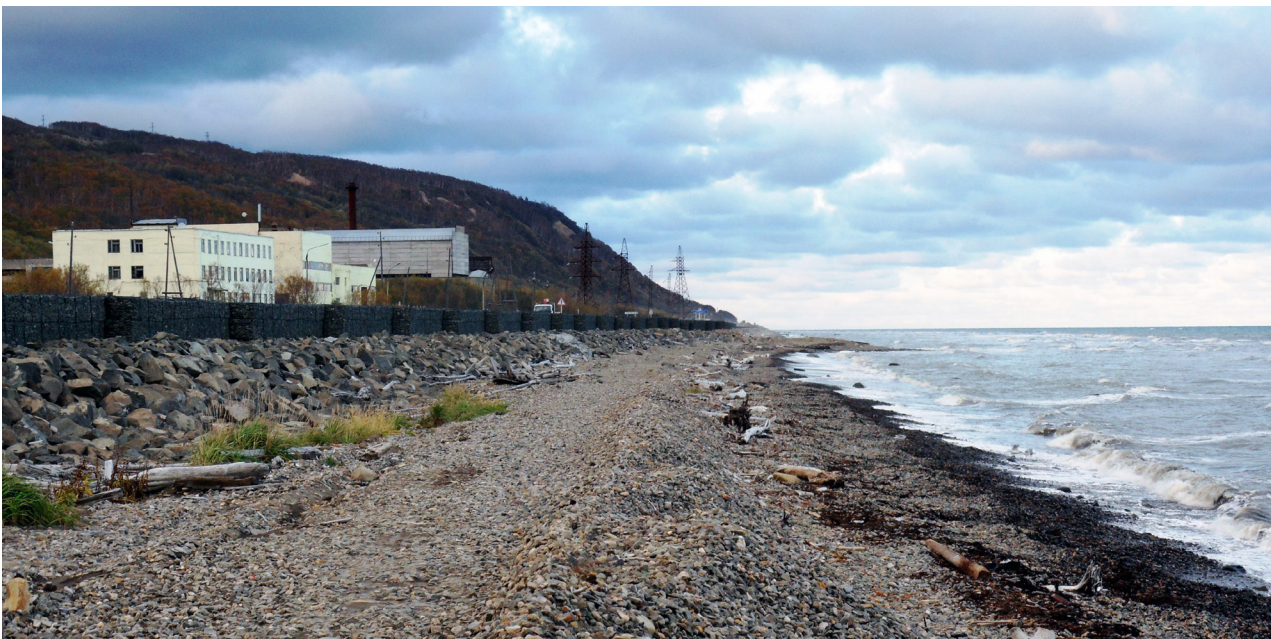
Fig. 1. Coastal shore erosion protection (Sakhalin Island). The lower part of rock revetment is covered by artificial pebble sediments, the gabion wall at the top is a splash protection to prevent the formation of ice on the road during the cold period. Photo by V. Afanasiev
